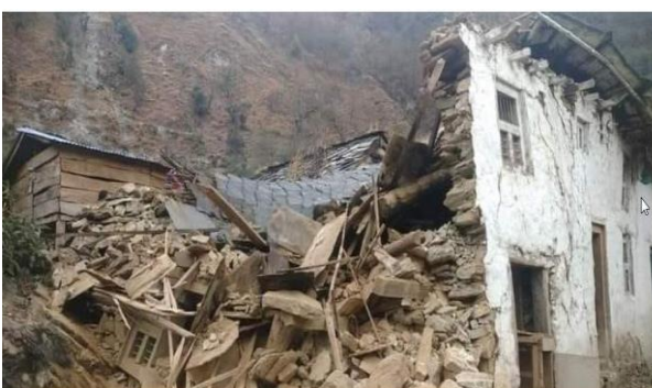
Building damaged during Earthquake of Jan 24, 2023 in Bajura District
